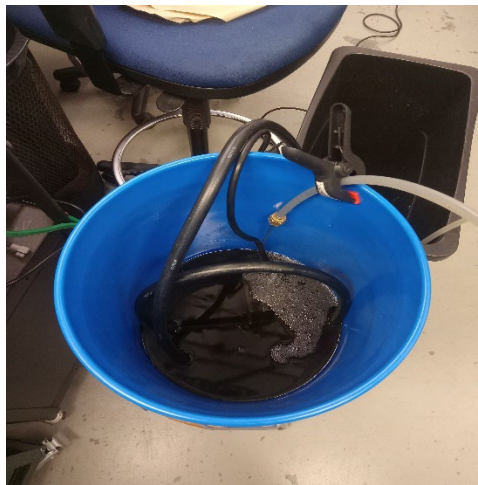
Fig 1. Bucket containing 1:1 solution of Rydlyme and water. The output tube is displayed facing into the bucket as part of the closed-loop descaling system.
